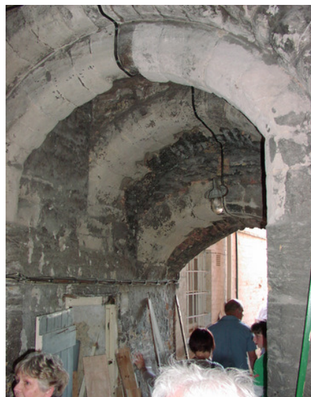
The triple-arch Water Gate is the most ancient structure in Bridgwater. Dr Cattermole deplored its present state—a cluttered alleyway sporting a blue plaque beside a derelict pub in West Quay—and urged everyone to email their dismay to kerry.rickards@sedgemoor.gov.uk .
