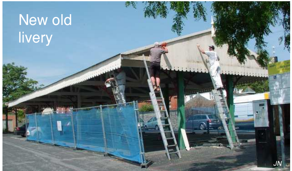
Martin Godfrey's bright idea to move the disused railway-station canopy to Glastonbury's main town-centre carpark won the Conservation Society second prize in the Civic Trust's Pride of Place competition in 1984. (Ian Rands, one of the society's volunteer labourers, tells of pulling millions of little nails.) After 30 years, the canopy had a thorough refurbishment this summer and now sports the authentic colours of the Somerset and Dorset Railway. Photographed at work are (from left) Mike Carter, Nick Payne and Nigel Petvin of J. Bailey & Sons, Wells.
