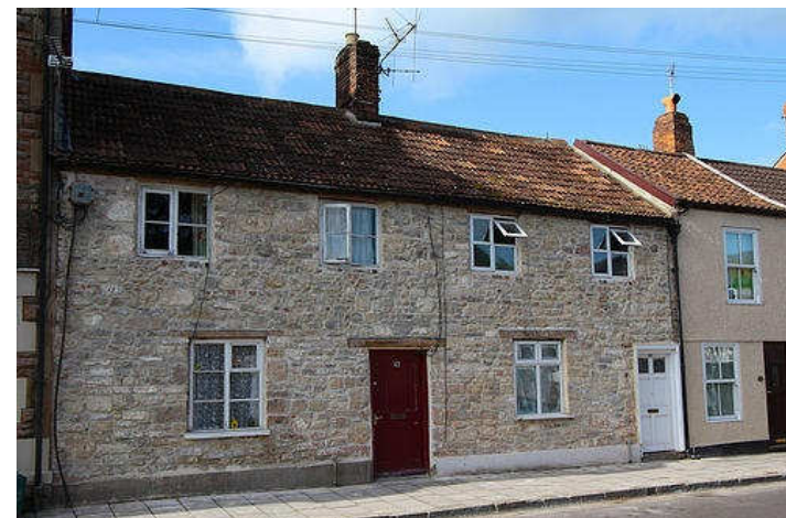
With render removed to reveal the Abbey stone from which they are built, the houses at 43 and 45 Benedict Street gain character.
