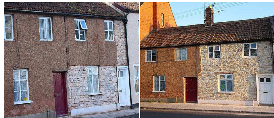
A lorry accidentally knocked drab pebbledash off the right of 45 Benedict Street, whereupon the owner and his neighbour stripped it all off to show the Abbey stone of their 17th-century cottages.
